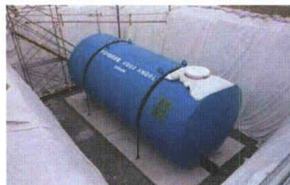
Earthquake-resistant, fire-safe water tank (Fukushima Daiichi Nuclear Power Station)
